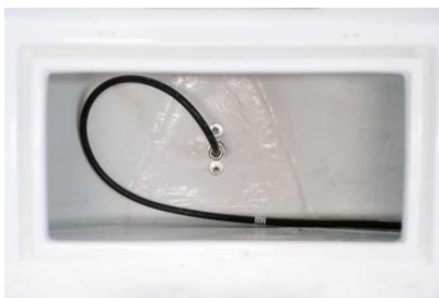
The new pod drive sticks up in the old motor room with a cable to the Lithium batteries, the control unit and the throttle. Foto: janajulian.com
